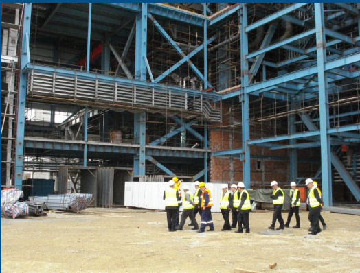
"Stanari Mine and Thermal Power Plant"
